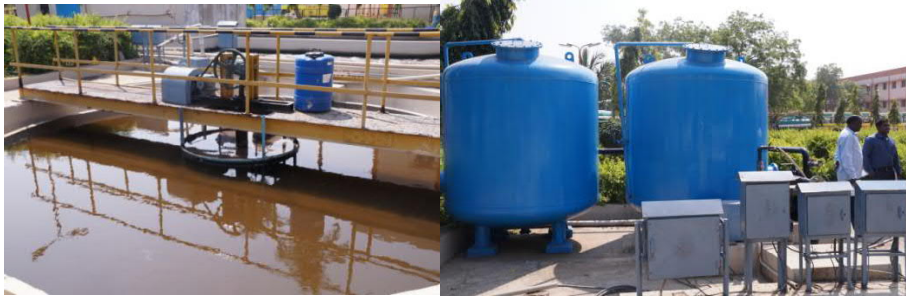
Fig. 7.2: Sewage Treatment Plant
