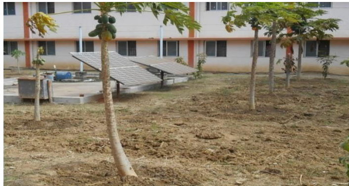
Fig. 7.3: Solar Power Plant
